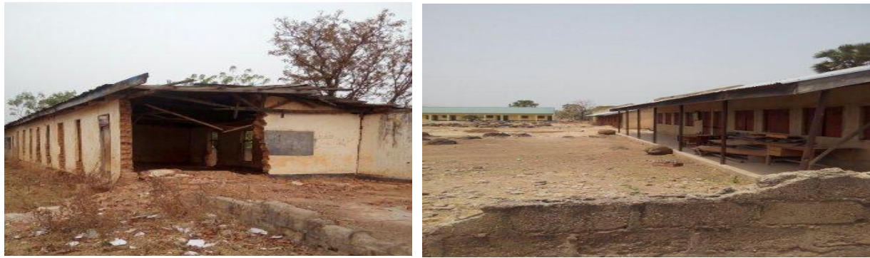
Plate 1: Dilapidated structure of LEA Primary School Bakin-Ciyawa and GSS Kwalla
